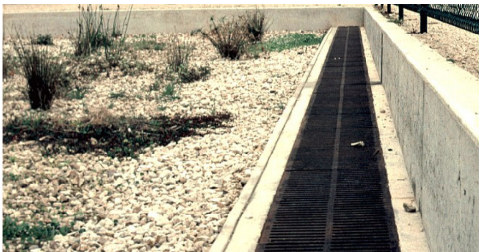
Infiltration bed with overflow grate and pipe
