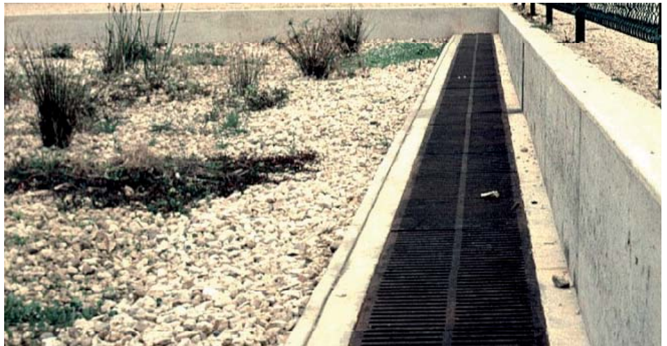
Infiltration bed with overflow grate and pipe
